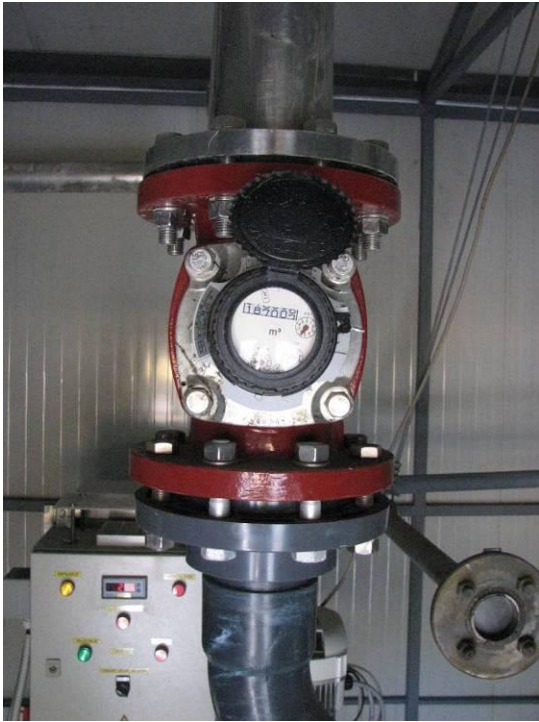
Figure 2. Flow meter on SOB-2 well.
